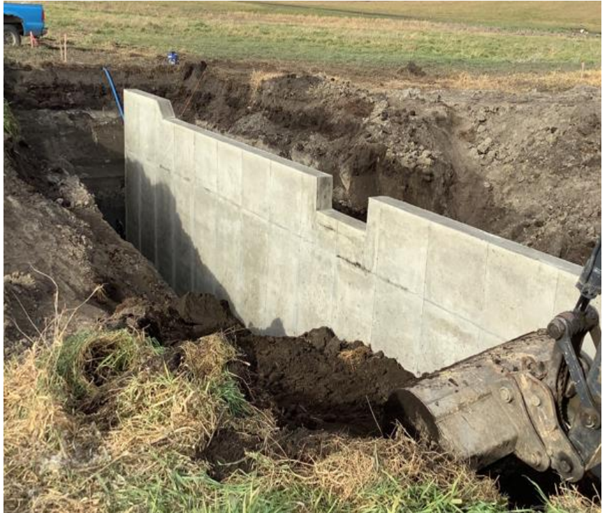
CD 61 storage and treatment wetland weir structure
