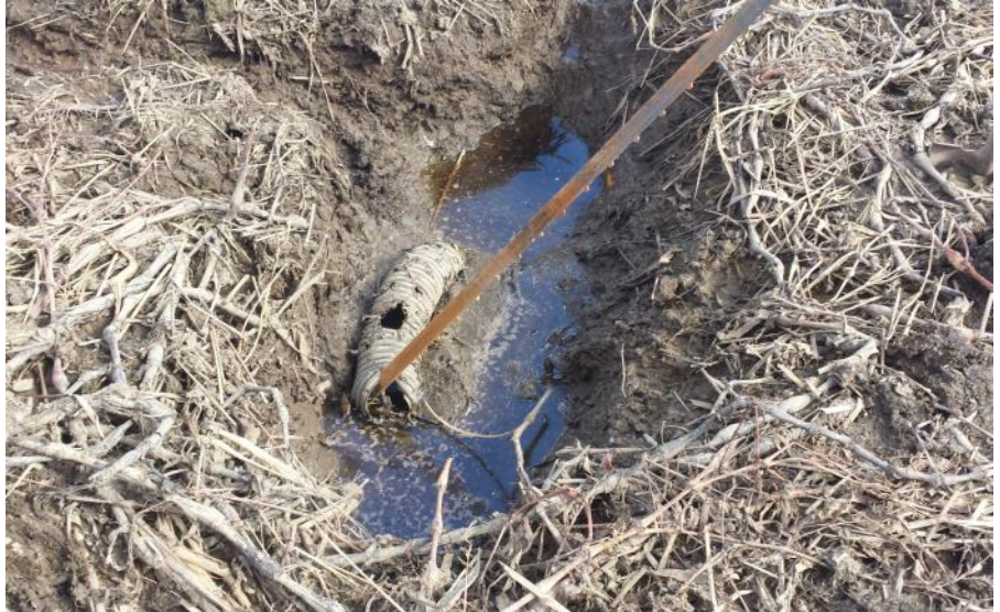
A WCA violation site where a landowner installed tile in a wetland.
