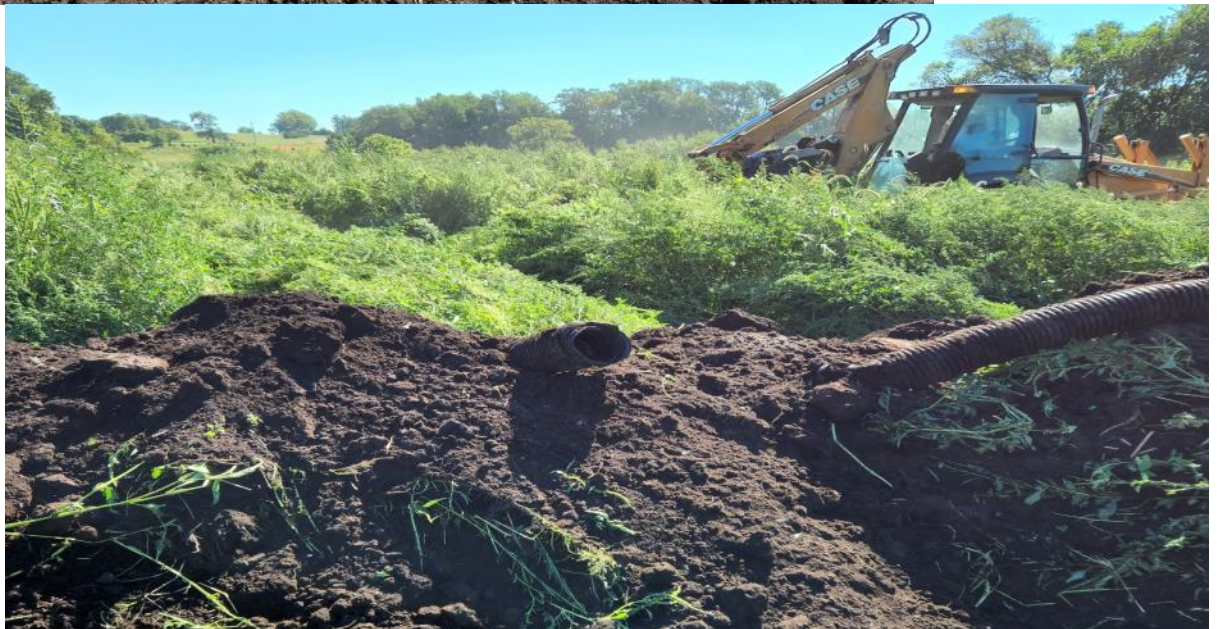
Tile Break completed to stop any future drainage from a wetland basin.
